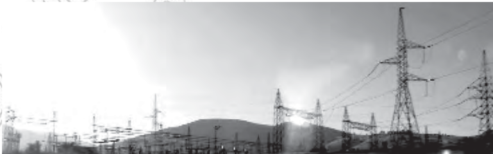
High voltage power lines and pylons
